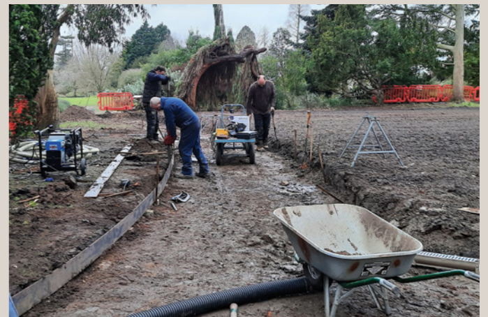
Above: Preparations for a new path from the main lawn to Middle Walk. Below: New path March 2021.
